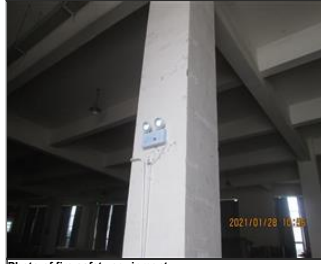
Photo of fire safety equipment Emergency lighting test.JPG
