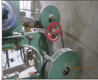
Photo of non-conformity NC Pulley guard was not installed completely.JPG
