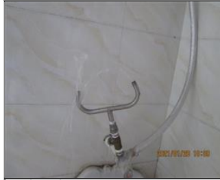
Photo first aid facilities Eyewash equipment.JPG
