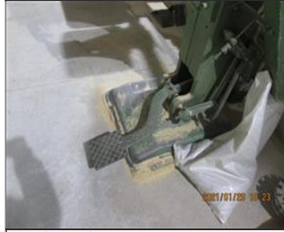
Photo of non-conformity NC No protective cover.JPG
